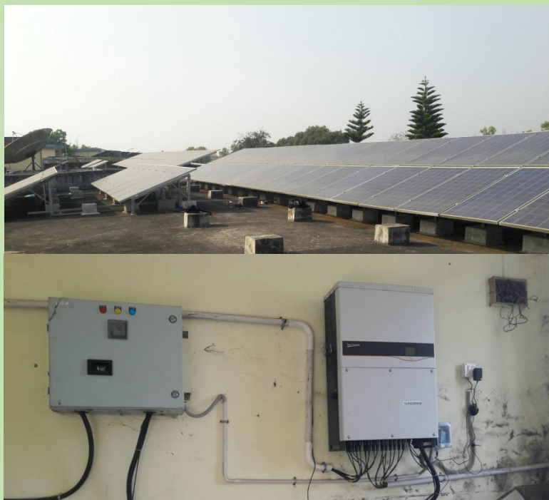
Fig 4: Use of solar power panels in TU Campus
